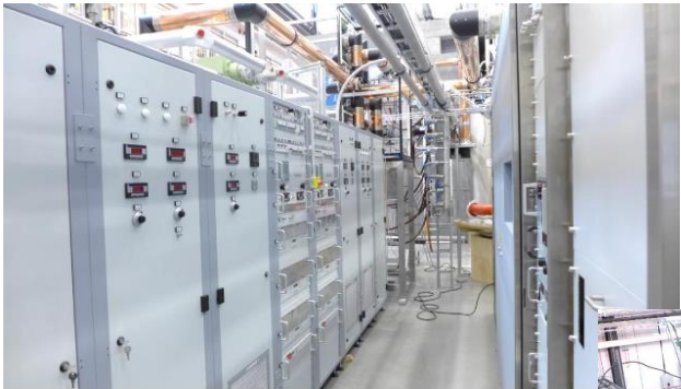
Power Amplifiers RF Distribution System
