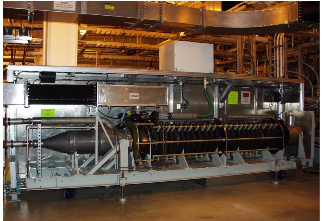
352-MHz/1.1MW cw klystron inside radiation shield enclosure
