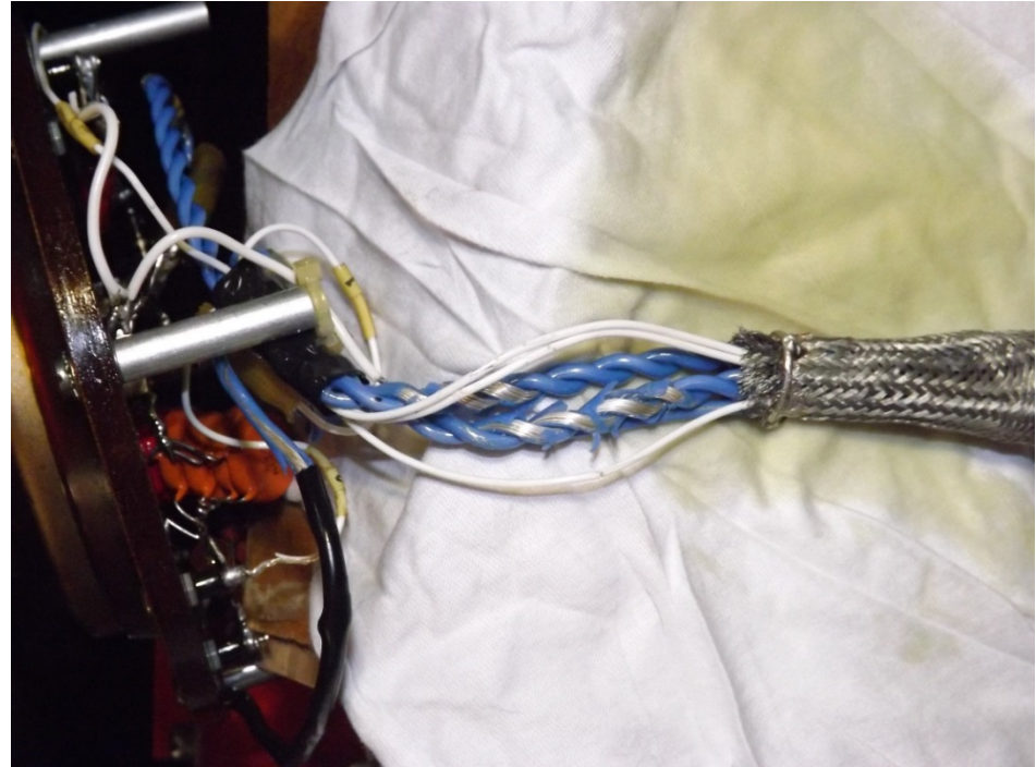
DAMAGED INSULATION ON WIRING LEADING TO TETRODE SOCKET
