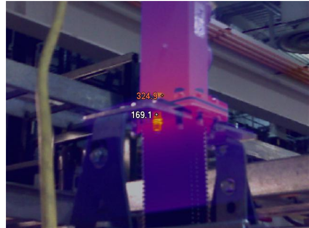
HOT FLANGE BOLT DUE TO IMPROPER TORQUE ≈ 2kW cw
