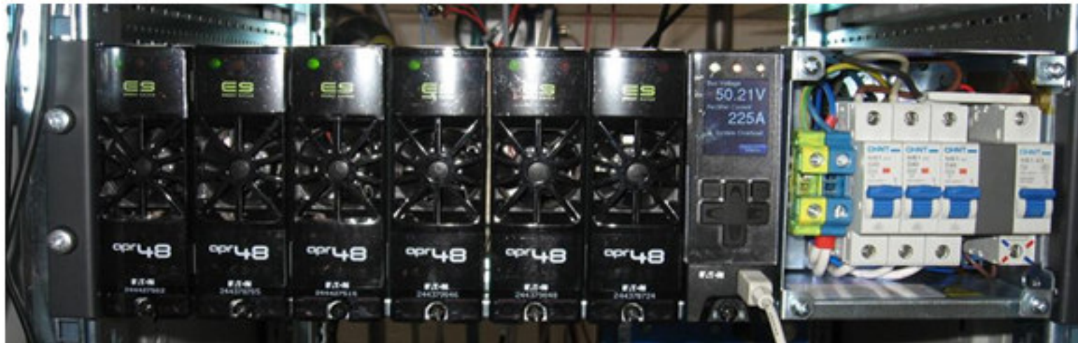
High efficiency (96%) 230 V ac / 50 V dc power converters
