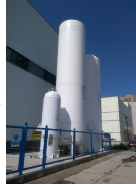
Buffer Tank & Impure Gas Tank & Liquid Nitrogen
