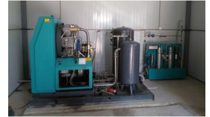
23m 3 /h Recovery Compressor
