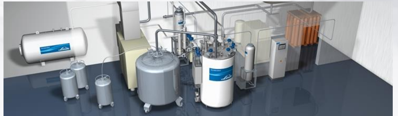
Linde liquid He production and recovery system - linde-engineering.com
